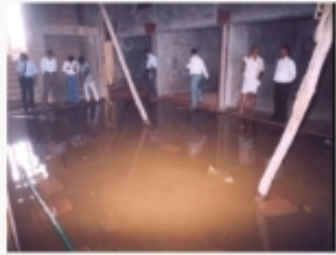
Stagnant water in ground floor
